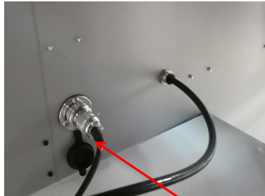
Vacuum pump power supply
